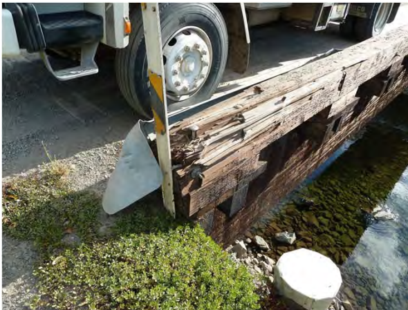
Figure 1-7: Damaged delineator and curb rail.
