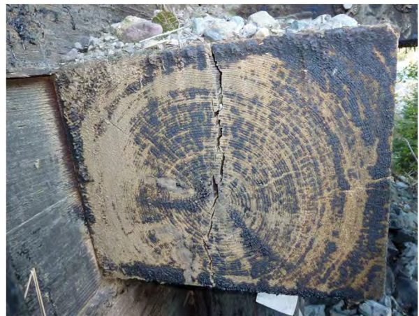
Figure 1-16: Check in woods end cap beam.
